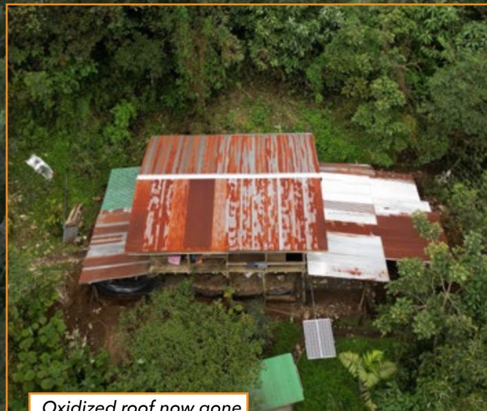
Oxidized roof now gone
